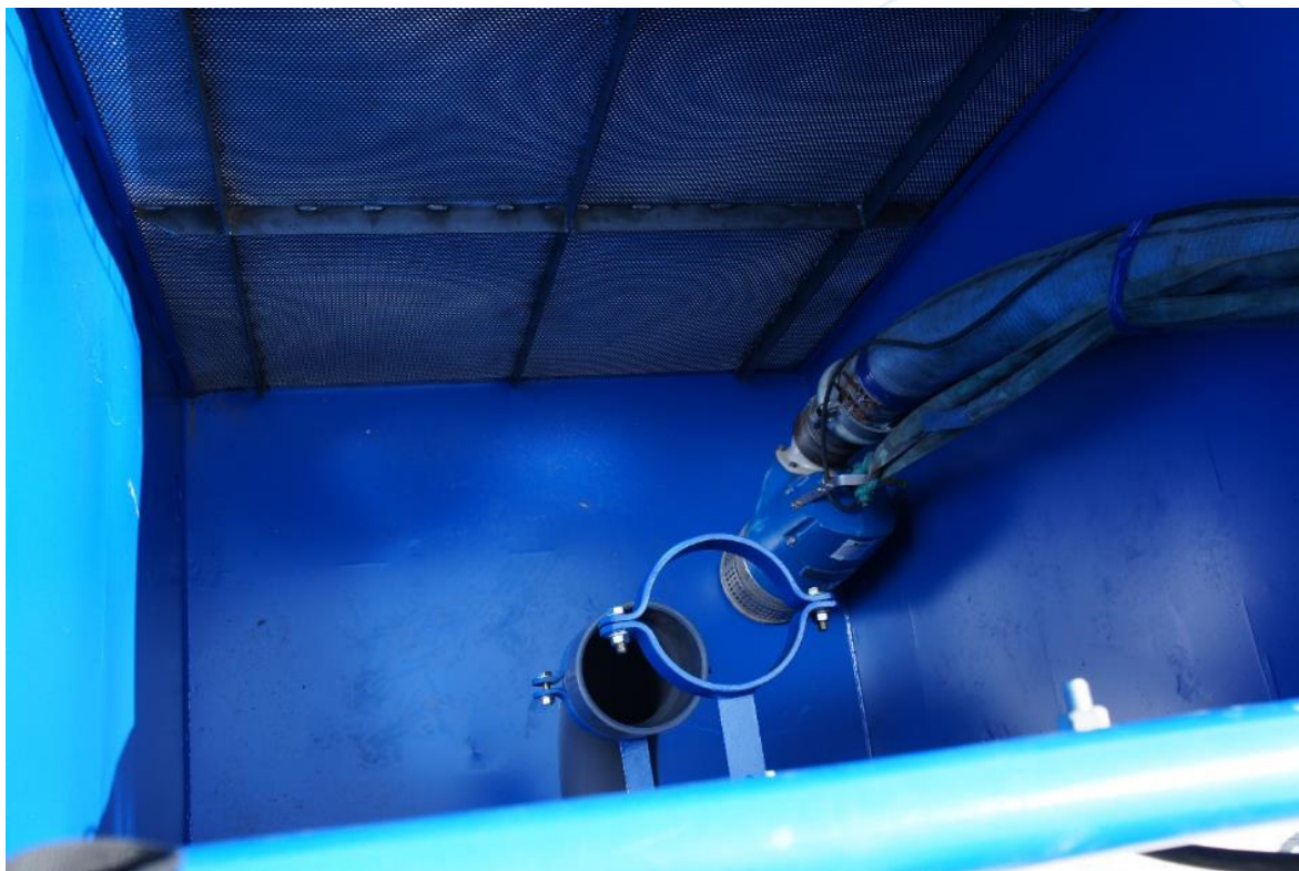
Figure 11. View into high water tank with mount for intake structure and pump for water supply
